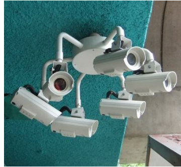
Fig. 7.6: CCTV cameras in a metro station.
